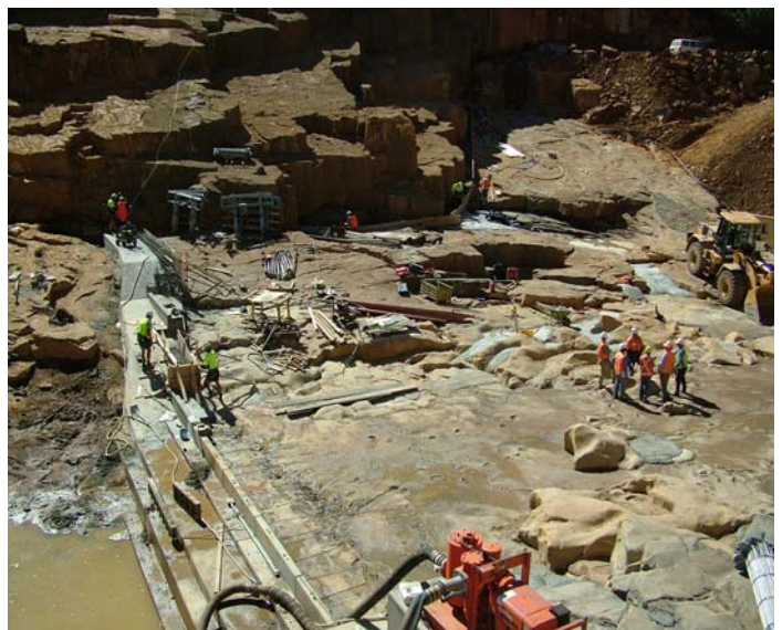
Above: Cleared River-bed ready to pour concrete with first pre-cast concrete blocks form-work in place.
